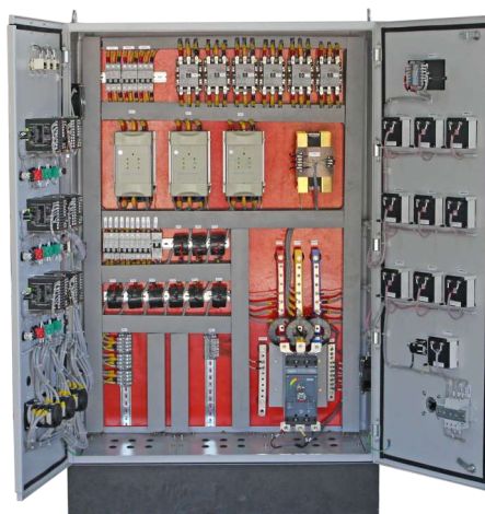
3-zone, 3-phase, SCR heating control panel internal view with bypass facility Type of load : Transformer (primary) Capacity : 270kw Application : SS wiring drawing annealing furnace
